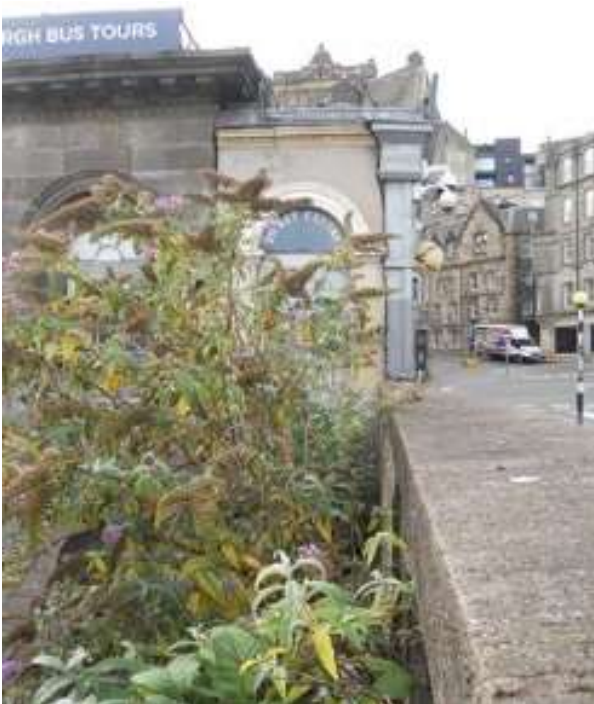
Buddleia on South Bridge and Waverley Bridge.
